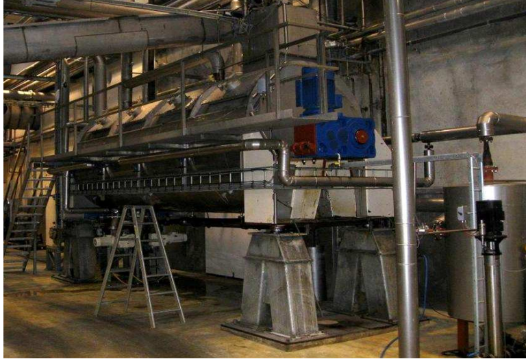
Super-cooker WHSC 1700 erected at DAKA in Denmark for pre-heating of raw materials
